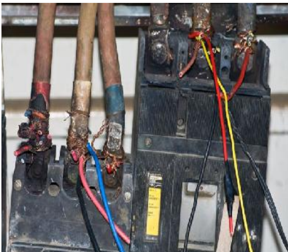
Figure4 Tampering of energy meters [7]
