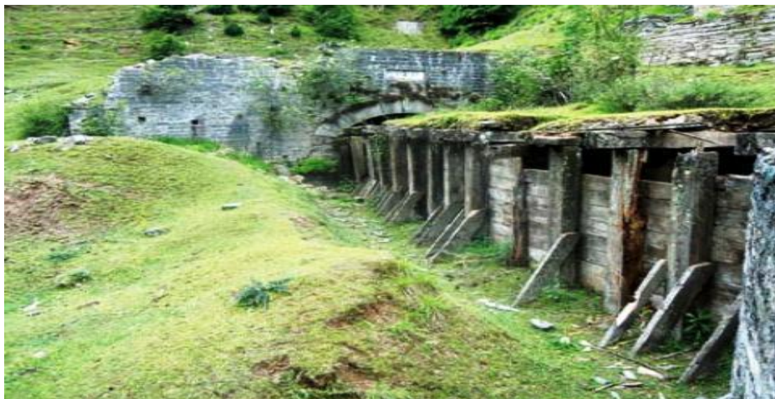
Figure1 Mohra hydroelectric plant [2]
