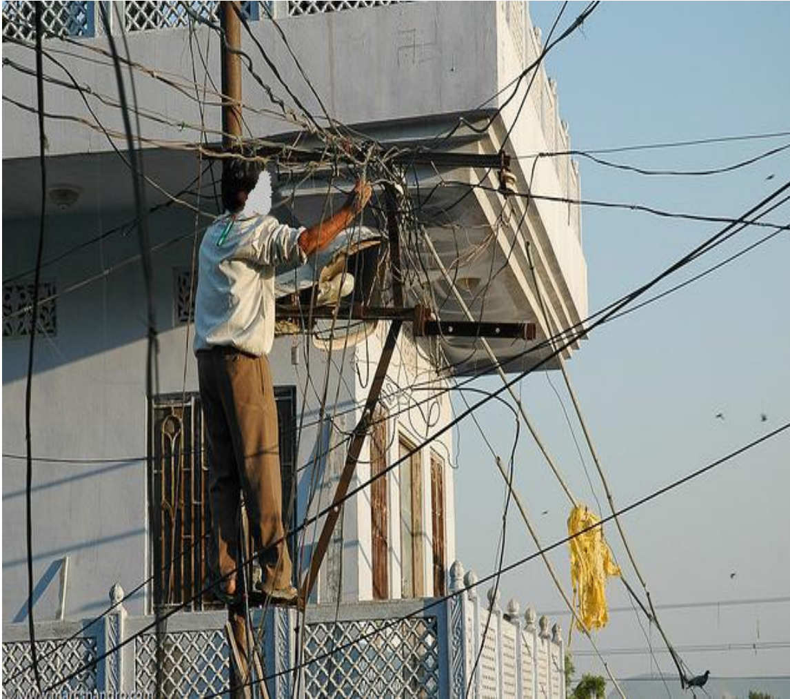
Figure5.Tapping on electrical line [8]
