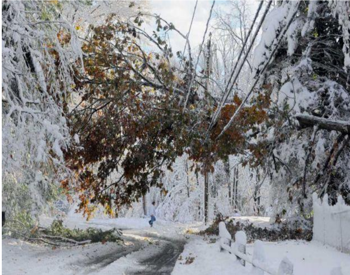
Figure 6 damaged distribution lines due to heavy snowfall [10]
